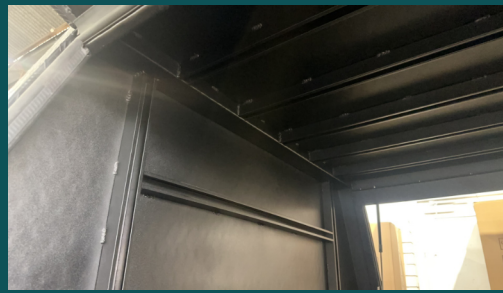
Internal unistrut reinforcing
